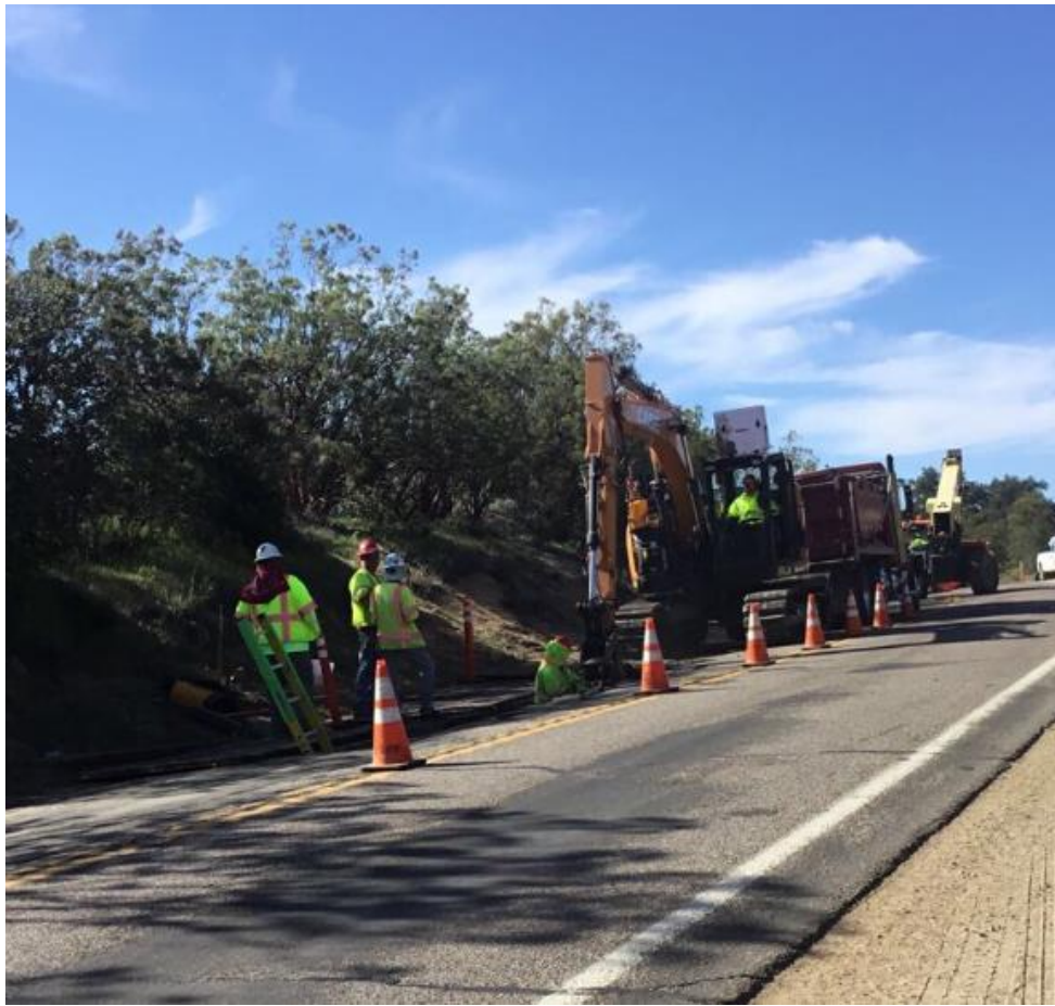
Photo 1: A Cultural Monitor was observed monitoring trench excavation along C449 in accordance with the HPMP and APM CUL-04.
