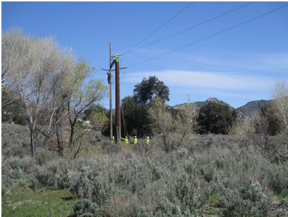
Photo 4: Construction crews were observed conducting overhead work (hanging travelers) at Pole Z40968 (TL 6958) in preparation for wire stringing. SWPPP BMPs (silt fencing) were observed in good condition in accordance with the MM HYD-1.
