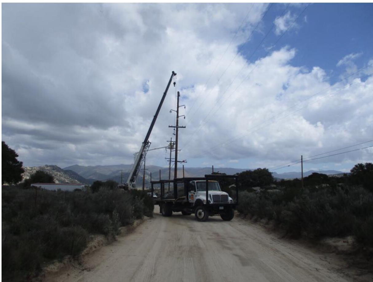
Photo 3: Construction crews were observed repositioning 69 kV lines on an old pole after spreading wire and installing a new pole at Z40792 (TL 6958). Traffic flaggers were observed along Cameron Truck Trail to stop and redirect traffic when necessary in accordance with APM TRANS-02.
