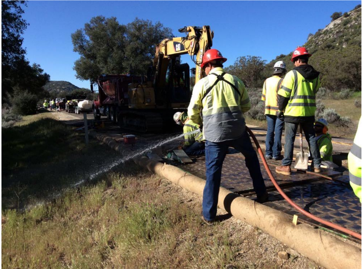
Photo 2: Hot work (using a torch to cut welding debris off steel plates) was observed along the trench at C449. A Dedicated Fire Patrol was observed wetting down the surrounding area and staging a complete set of fire tools in accordance with the CFPPP Fire Matrix for the day's fire conditions (PAL C on CNF land).
