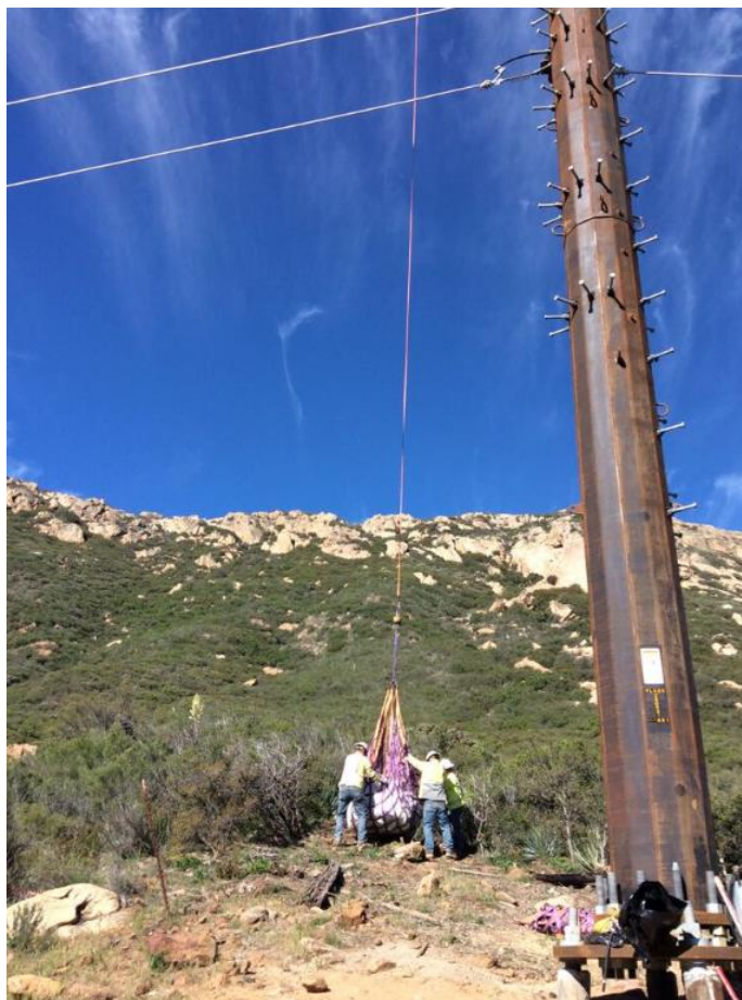
Photo 6: Helicopter external load operations were utilized to remove erosion control BMPs at Pole Z40421 (TL 629C). At the Buckman Springs Fly Yard, a water tender was observed applying water to the surface to minimize dust emissions from rotor wash in accordance with APM AIR-02.
